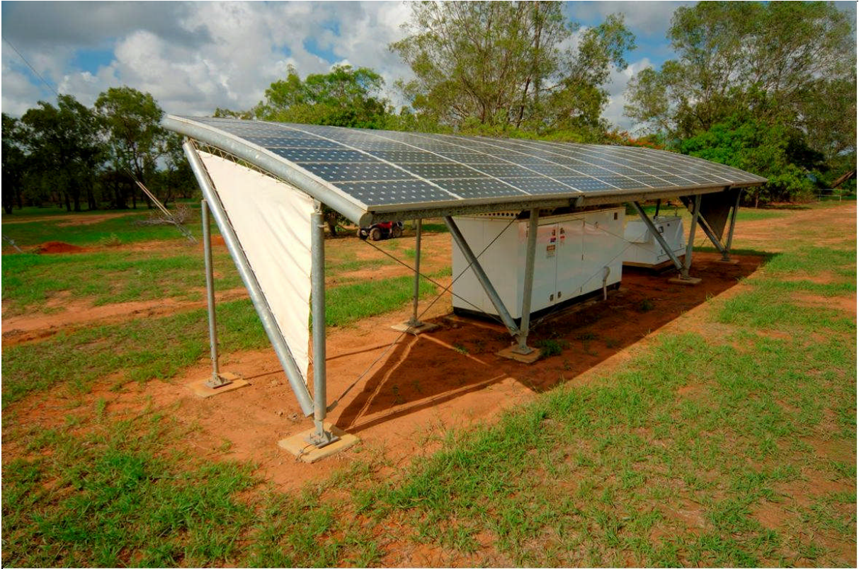
Solar-diesel hybrid station [Picture ERGON, Australia]
