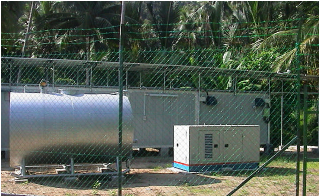
Solar Hybrid Power Station [TNB, Malaysia]
