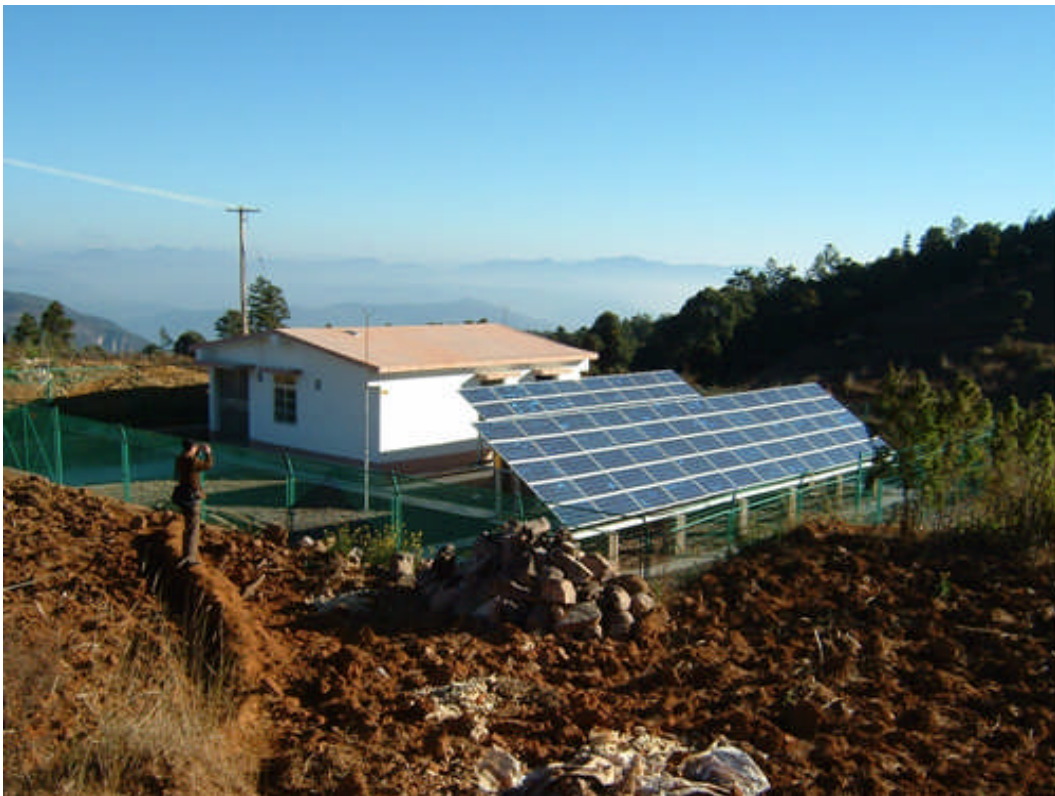
Large PVHybrid system with diesel genset [SMA Technologie, Germany]
